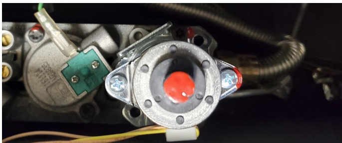
Figure 13.eee LP pressure regulator on a Full Load
